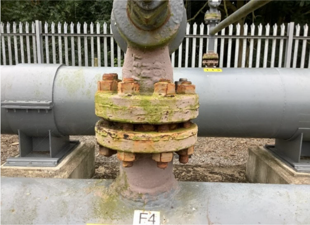
Figure 2: One of several valves at [REDACTED] requiring patch painting associated with UID [REDACTED]
